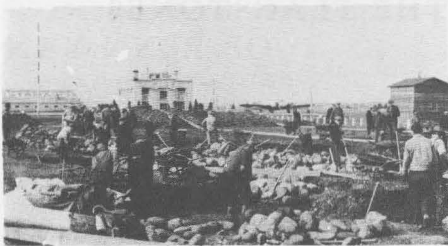
Felts Field Airport, Spokane, Spokane County, Washington. W.P.A. workers are shown constructing a new hangar and administration building.
