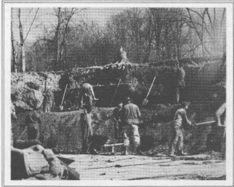
At left, WPA workers shelving banks of the new Fall Creek channel, Millersville, Marion County, Indiana.
