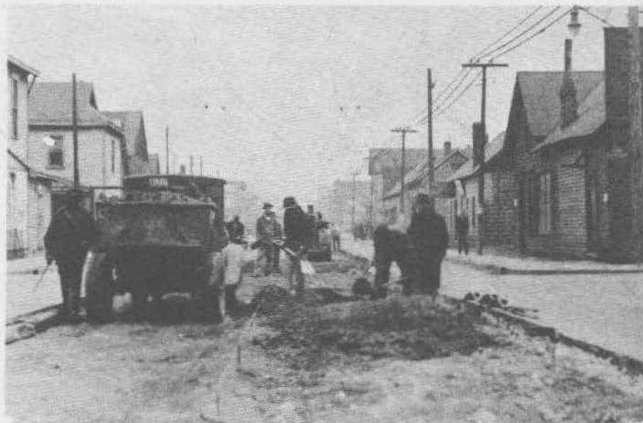
Repair and construction on West Michigan Street in Indianapolis, Marion County, Indiana, by WPA workers.
