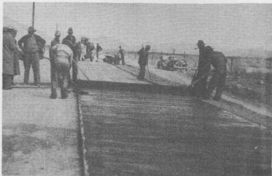
Road paving in Cochise County, Arizona, WPA workers are shown laying a pre-mixture of emulsified asphalt.
