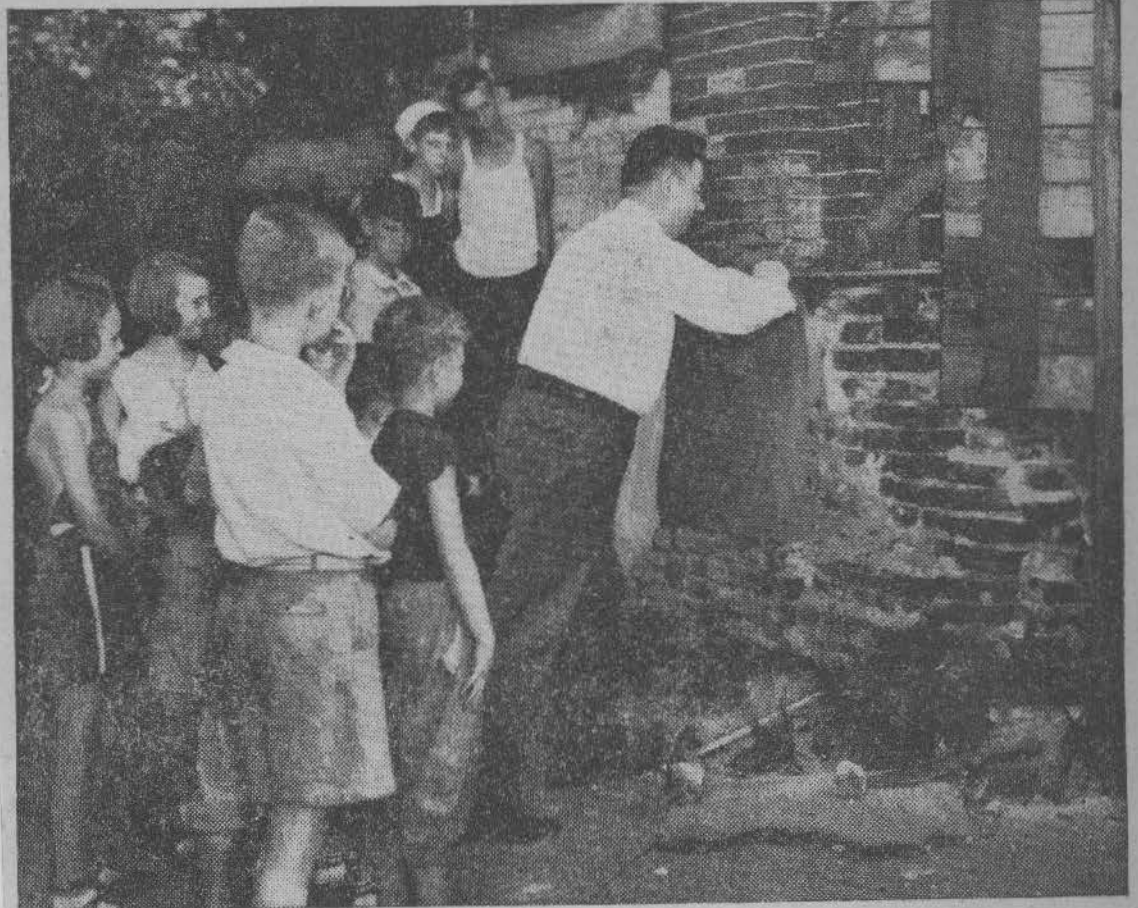
Sheriff Hamilton personally began demolition of the old car barn at Sumac Street and Rochelle Avenue today under the approving eyes of neighborhood youngsters. The structure will be replaced by a park and playground
