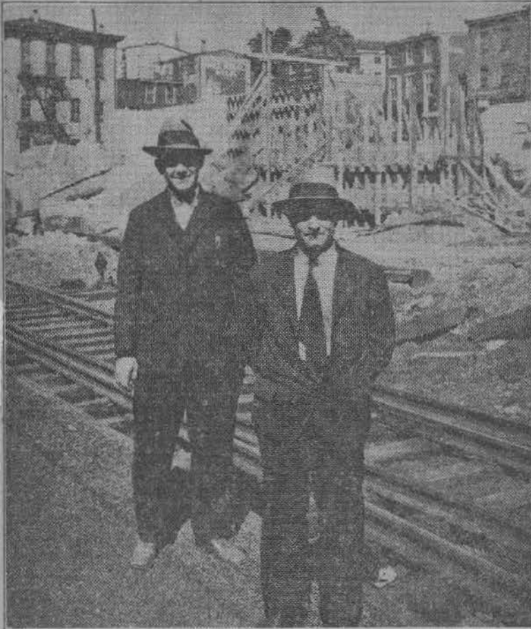
Presenting to our readers a photograph of Adolph Jafolla, (right) and William Mark, the contractors who are making rapid progress on the erection of the Reading Railroad Company's elevated structure through Manayunk. They are here seen, standing on the site of the new passenger station, which will be erected between Carson and Gay street. These men, by what appears to be a miracle, are now fifteen weeks ahead of the schedule on what was supposed to be a twenty-month contract.
